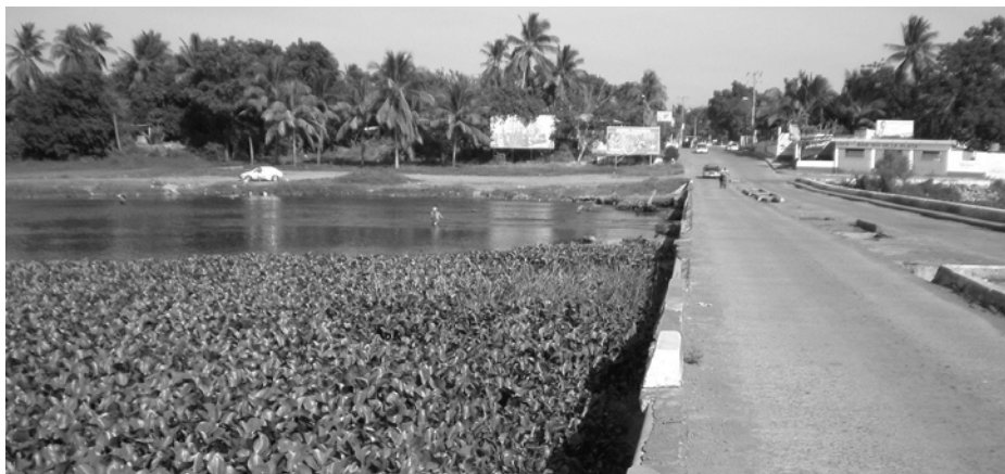
Figure 1: Bad conditions of the bridges close to the mouth of the River Actopan
