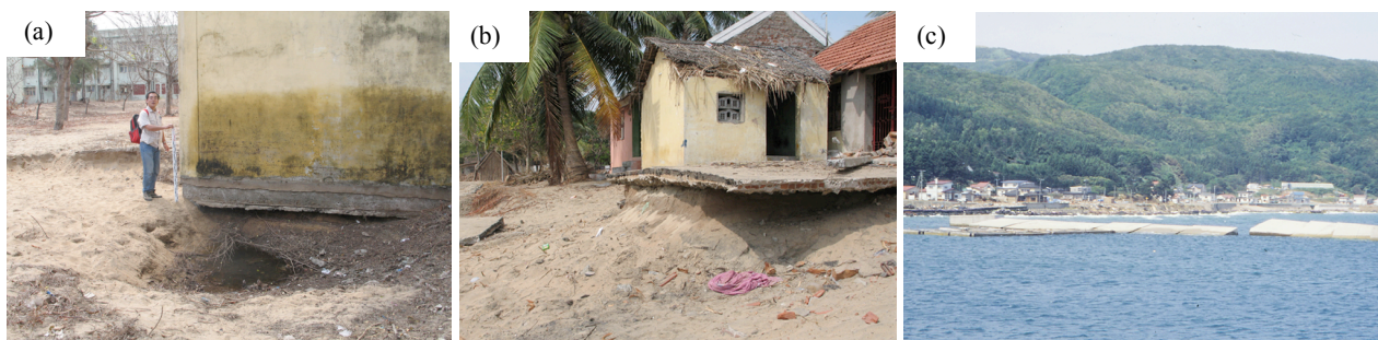
Figure 1. Typical scour holes at building foundation: a) approximately 1.5 m deep in India, 2004 tsunami (photo by Yeh); b) 1.4 m deep in India (photo by Yeh, PI); c) foundation failure of the breakwater by the tsunami (Okushiri, Japan, 1993; photos by Yeh).
