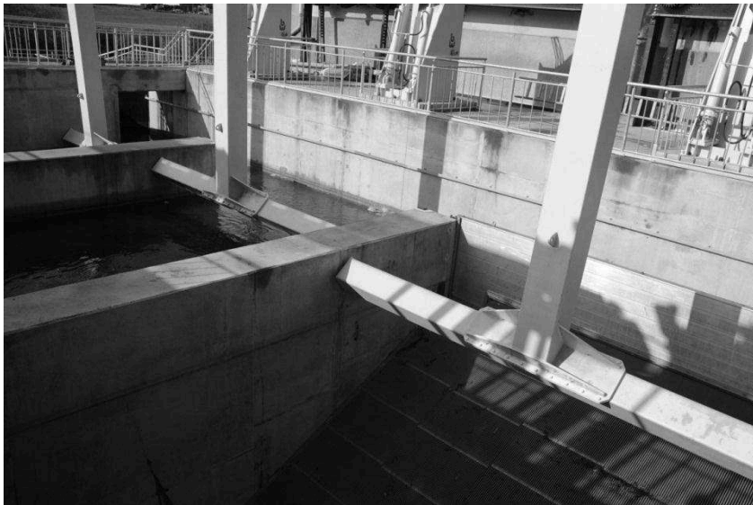
Figure 6. Three-bay bar screen array with flushing channel in the back.
