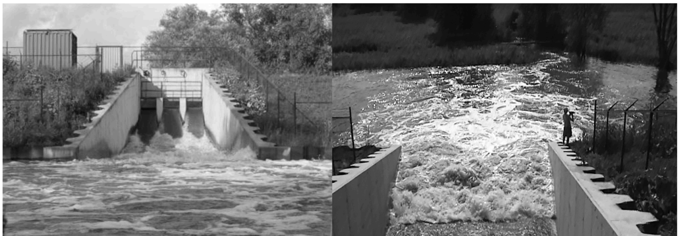
Figure 6. Energy dissipation and aeration of water flowing into FCA-CRT Lippenbroek (left: view from polder towards inlet sluice ; right: view from inlet sluice towards polder).
