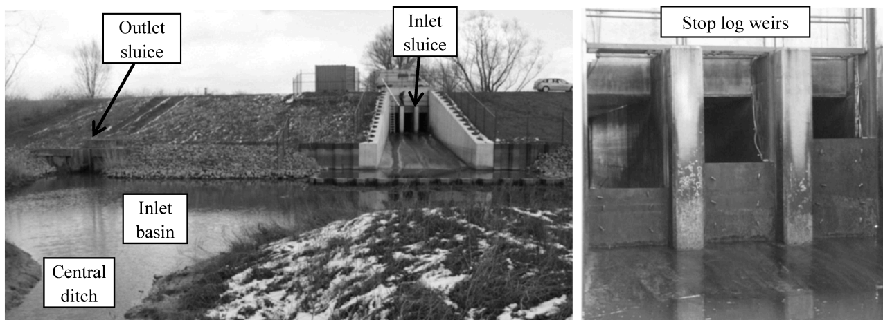
Figure 4. View from polder upon inlet sluice and outlet sluice of FCA-CRT Lippenbroek (left) and upon stop log weirs at downstream end of inlet sluice culverts (right)
