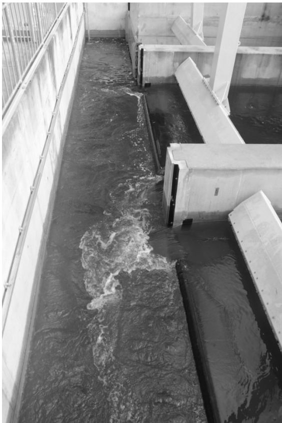
Figure 7. Flushing channel and surface bypass openings for salmon smolts in the top area of the fish protection screens.
