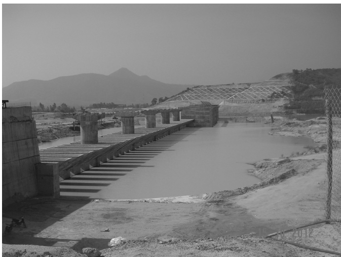
Figure 3. Von Phong dam (Vietnam) in-channel PK weir under construction (photo courtesy of Quat Dinh Sy).
